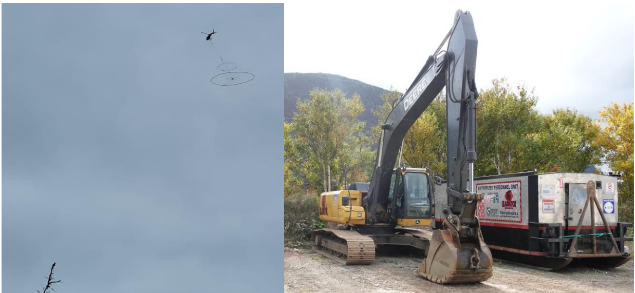
Figure 1: Heli-EM, Drill Rig and earthworks support vehicles mobilised at Skyline Copper Project
