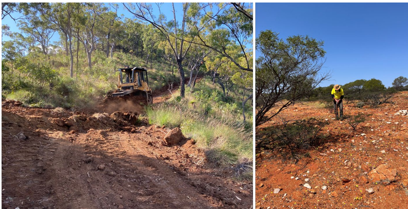
LEFT: EARTHWORKS AT MT SLOPEAWAY PROJECT, QLD OCTOBER 2022. RIGHT: PEGGING PROPOSED DRILL LOCATIONS AT YALGOO PROJECT, SEPTEMBER 2022
